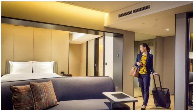
On entering a room at the Swissôtel The Stamford, Interact Hospitality turns on the lights automatically after sensing movement.
