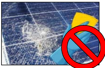
Do not clean broken PV panel
