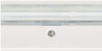
Emergency ExitSign Wireless, test button
