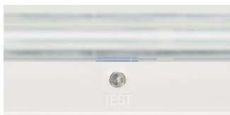
Emergency ExitSign Wireless, test button
